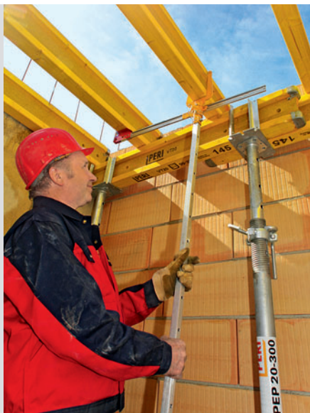
Fast and safe installation and aligning of the main beams with the Fixing Tool.
